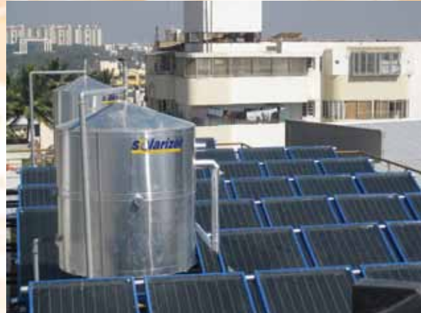
Baptist Hospital, Karnataka - 9500 LPD
