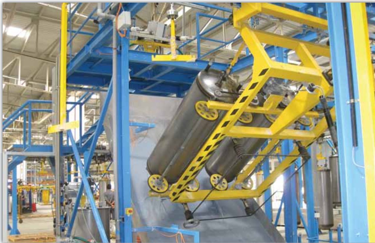
Enamel Coating Plant
