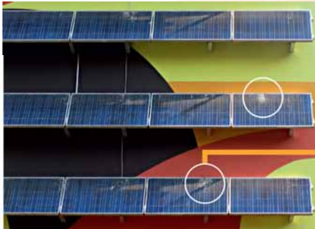
Example of installation which must be avoided: Performance loss due to shading in the morning hours and contamination of bird droppings.
